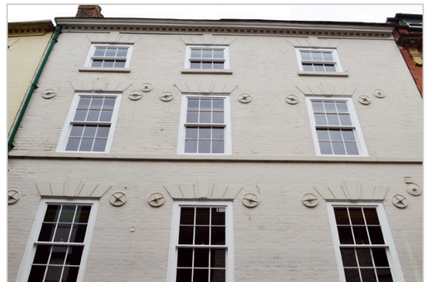
Grade II mid 18 th century. New box sash, single-glazed replacement windows with 19mm fine glazing bars with lamb's tongue internal profiles.
