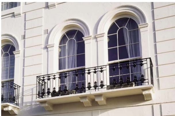
Grade II (1845). New round headed, box sash, double-glazed replacement windows with 17mm fine glazing bars with lamb's tongue internal profiles.
